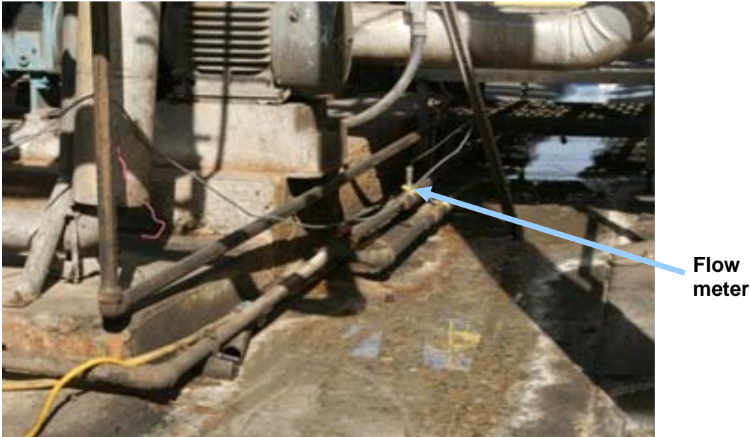
Figure 8 Flow meter installed on the steam condensate return line
