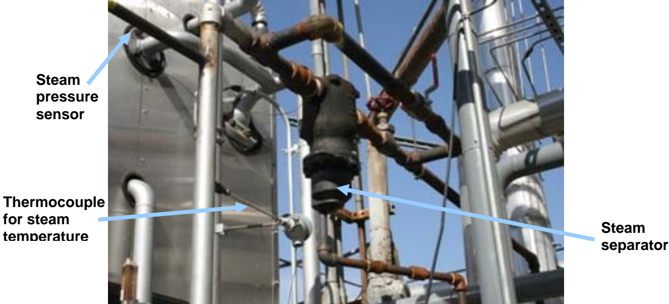
Figure 7 Monitoring equipment installed on the steam input line
