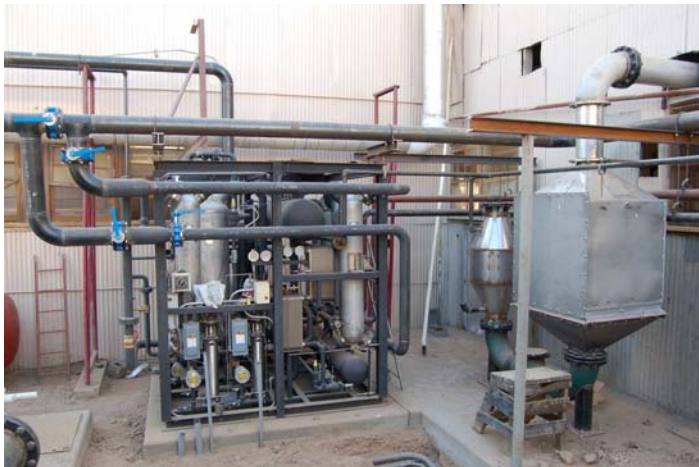
TC160 and one Heat Recovery Vapor Generator
